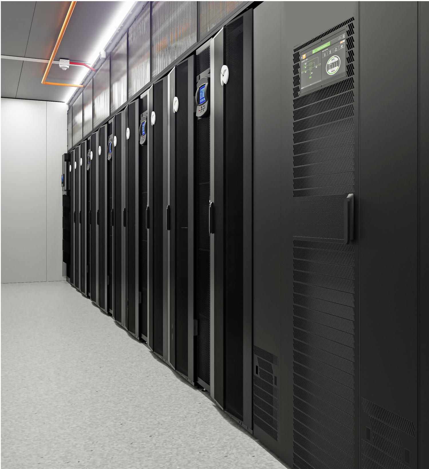
Interior view of Vertiv SmartMod
